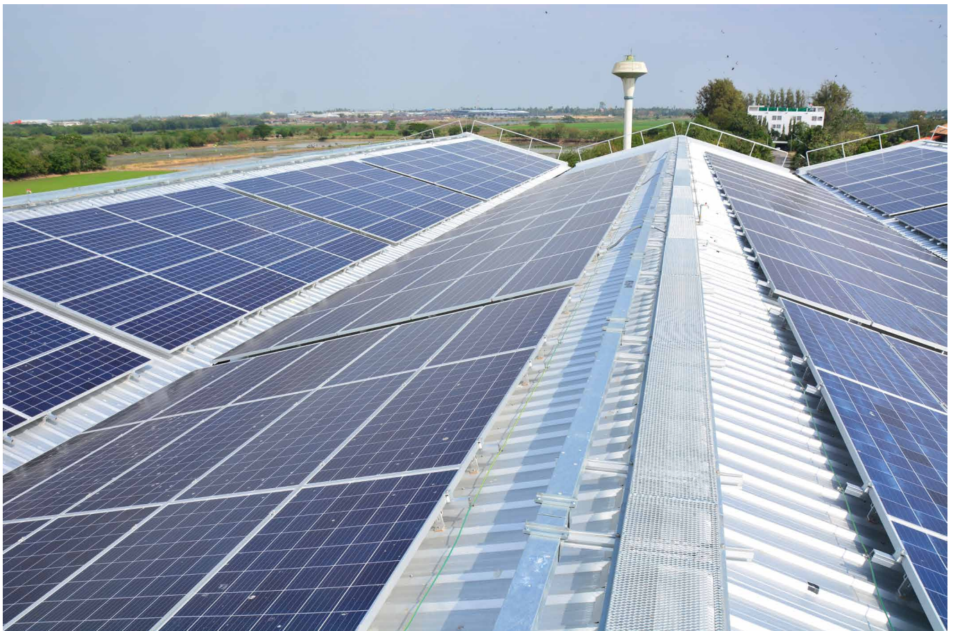
Rooftop solar photovoltaic (PV) system
