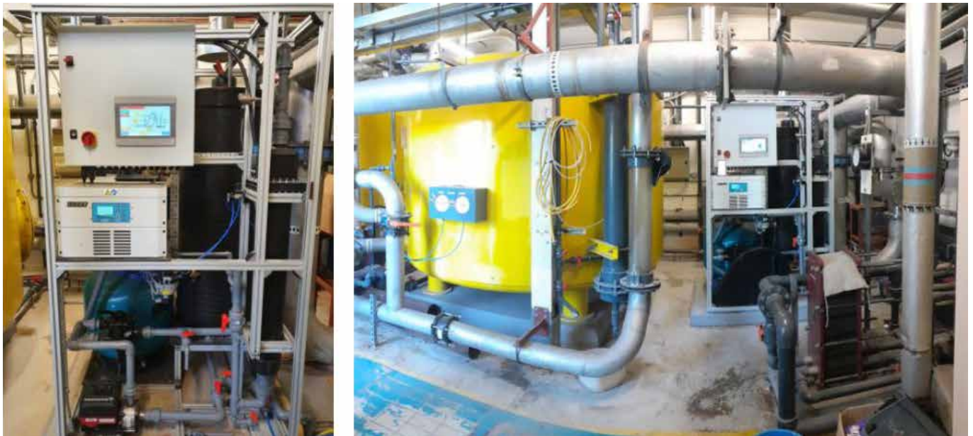
Backwash water recovery system
