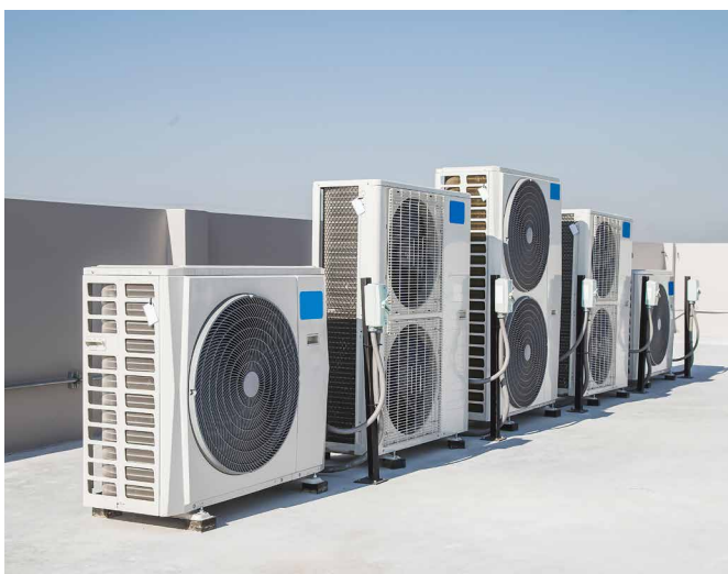
Rooftop heat pumps
